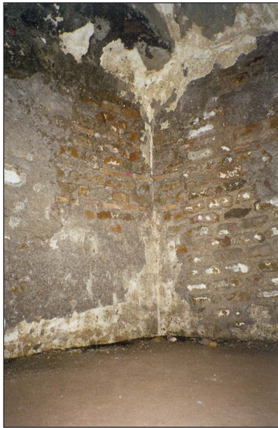
Figure 23. Detail of irregularly shaped barrel vault in m. (Photo: J. Dello Russo)
