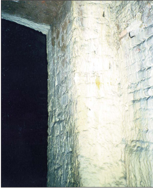
Figure 36. Doorframe and supporting piers around lucernarium L1 of ancient brick and marble fragments, with a thick white deposit of calcium from the water seepage from above. (Photo: J. Dello Russo)
