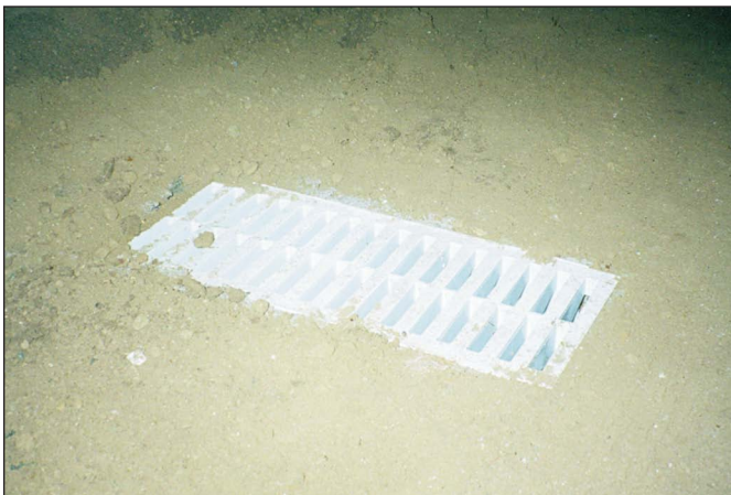
Figure 56. Installation of a grate in G1 to collect seepage from lucernarium L3. (Photo: J. Dello Russo)
