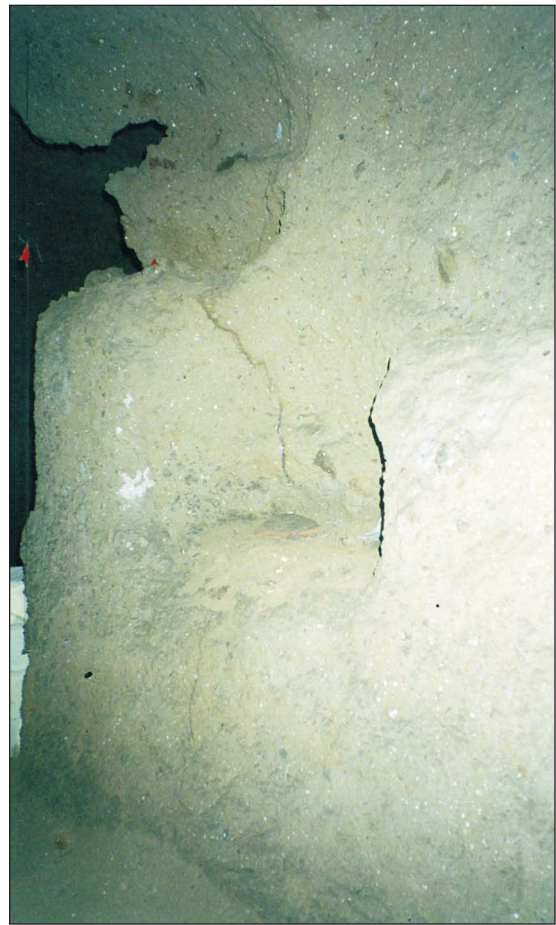
Figure 47. Original, fragmentary state of wall in D before reinforcement. (Photo: J. Dello Russo)
