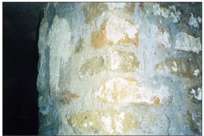
Figure 24. Detail of wall of tufelli and opus vittatum, traces of plaster, in m. (Photo: J. Dello Russo)
