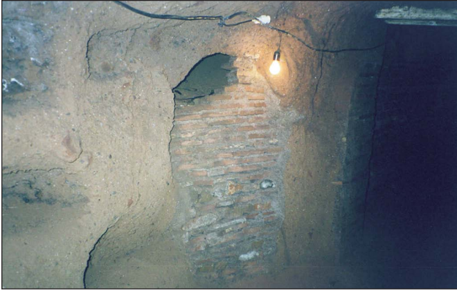
Figure 27. Loculi damaged by gallery opening, gallery in turn blocked by ancient brick wall (connecting galleries in m to G1?) (Photo: J. Dello Russo)
