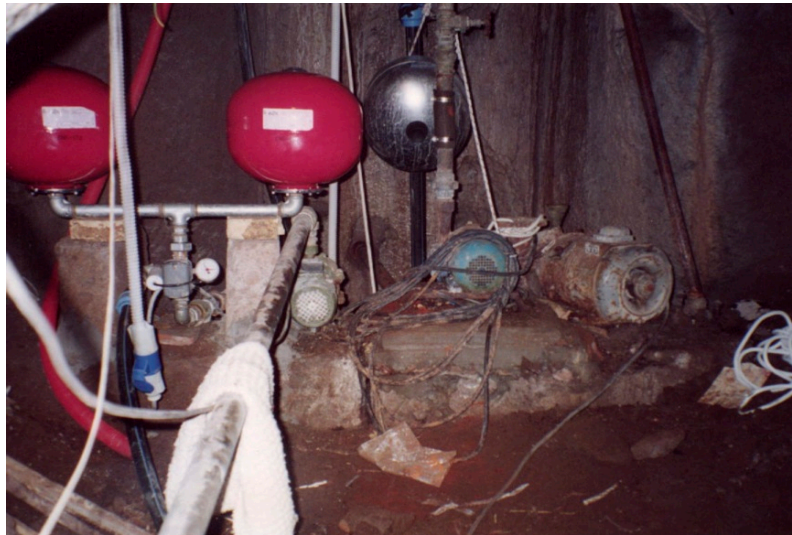
Figure 28. Newly installed water pump inside the quarry/well area. (Photo: J. Dello Russo)
