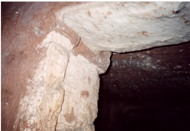
Figure 17. Detail of the marble doorframe of the cubiculum, showing calcium deposits over its surface. (Photo: J. Dello Russo)
